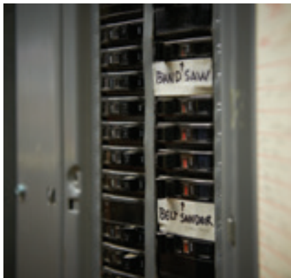
Label electrical components: 3M™ Masking Tapes ( pgs 57-60 )
