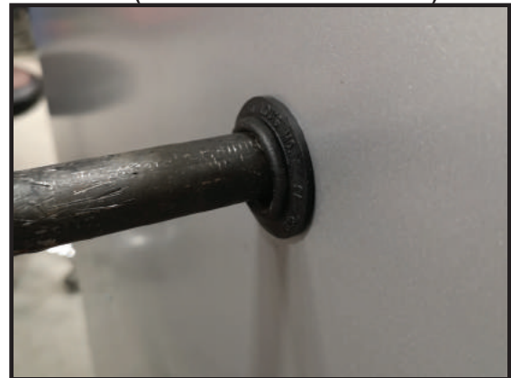
FIGURE 28 - FURNACE GAS PIPE CONNECTIONS (NOTE RUBBER GROMMET)
