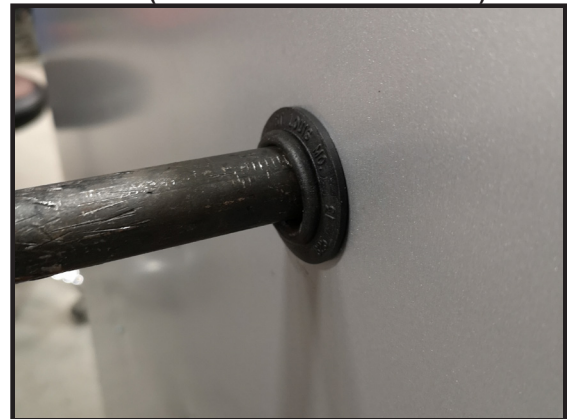
FIGURE 28 - FURNACE GAS PIPE CONNECTIONS (NOTE RUBBER GROMMET)
