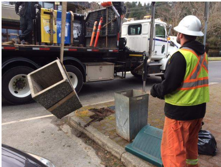
Bin replacements were staged over several weeks, completed using a crane truck
