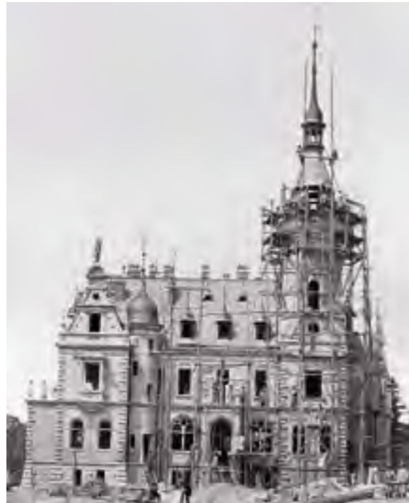
The construction of the family seat in Schwarzenbruck was begun in 1883; by 1885 the shell was complete.
