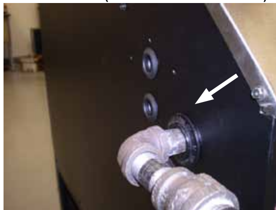
FIGURE 26 - FURNACE GAS PIPE CONNECTIONS (NOTE RUBBER GROMMET)
