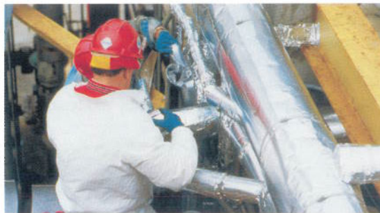
Installing the ceramic mat insulation on the complex conduit lines at Ashland's St. Paul plant was hastened by the ability to cut and fit the material with common tools
