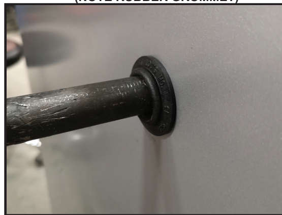
FIGURE 28 - FURNACE GAS PIPE CONNECTIONS (NOTE RUBBER GROMMET)
