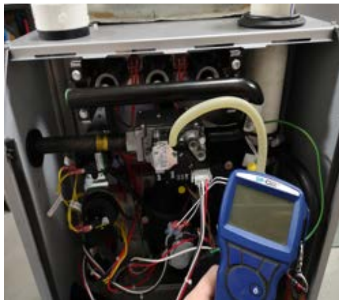
FIGURE 30 - MANOMETER MEASURING GAS MANIFOLD PRESSURE
