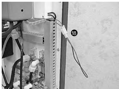
Level switch connector wire
