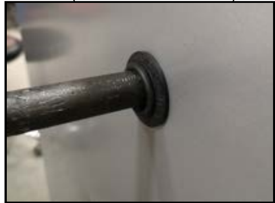
FIGURE 28 - FURNACE GAS PIPE CONNECTIONS (NOTE RUBBER GROMMET)
