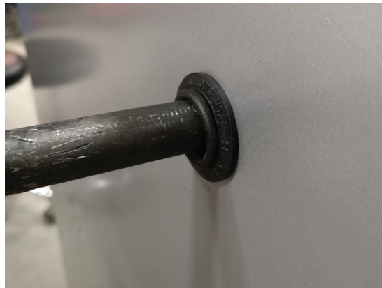
FIGURE 27 - FURNACE GAS PIPE CONNECTIONS (NOTE RUBBER GROMMET)
