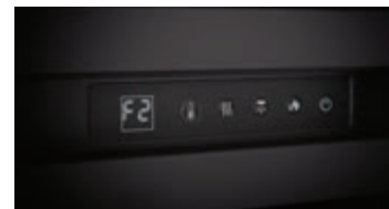
Control panel with white LED display
