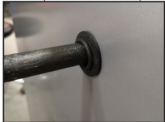
FIGURE 28 - FURNACE GAS PIPE CONNECTIONS (NOTE RUBBER GROMMET)
