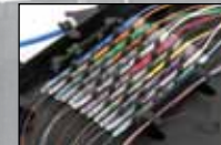
Room to splice inside (288 F capacity)
