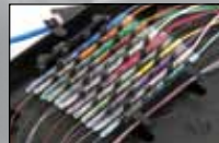
Room to splice inside
