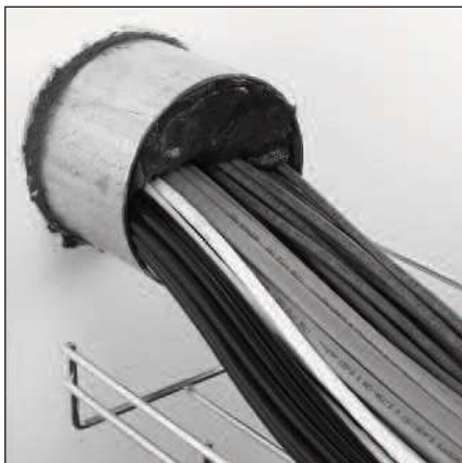
1. Existing conduit with cables. Remove firestop putty.
