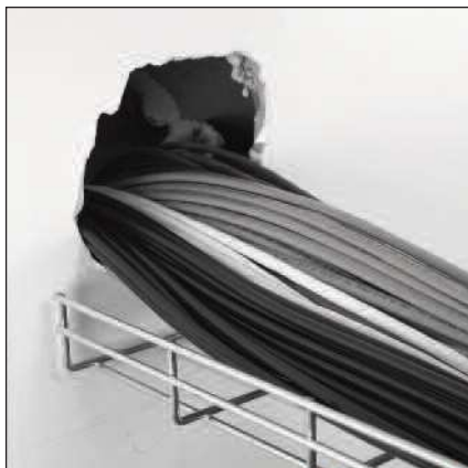
1. Existing hole with cables. Irregular hole cut.
