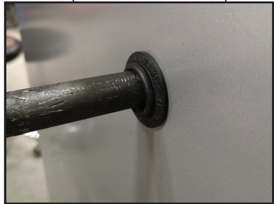
FIGURE 28 - FURNACE GAS PIPE CONNECTIONS (NOTE RUBBER GROMMET)
