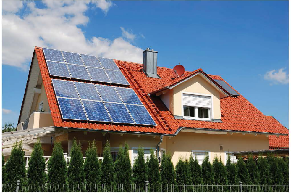
Solar panels on a roof harness sunlight to generate electricity for a building.
