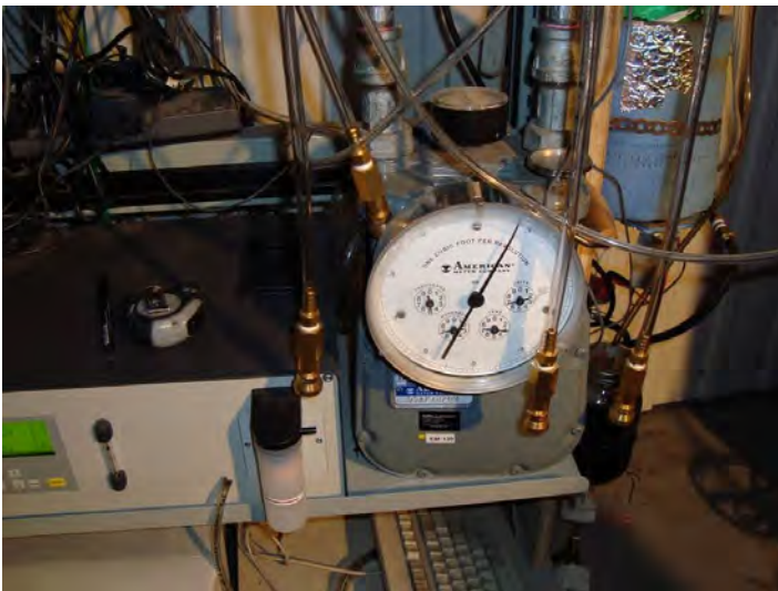
Picture 8 : Reference dry gas meter
