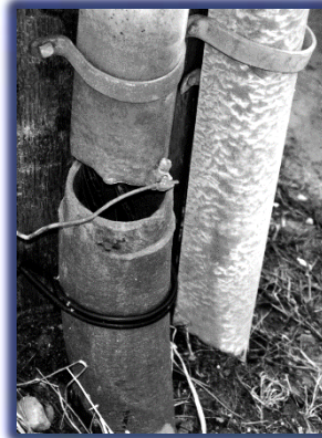
Steel U-Guard required grounding, strapping, and does not have belled ends.
