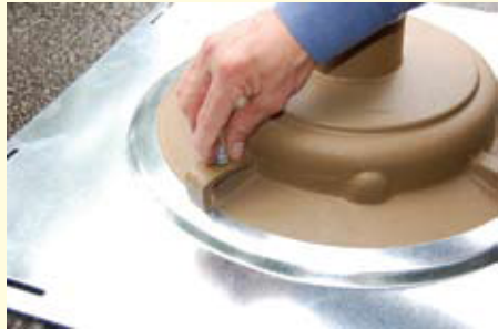
3. Bolt the 4 angled steel support buckets onto the roof drain until the deck plate is locked into place. (See -DPK Trim Kit)
