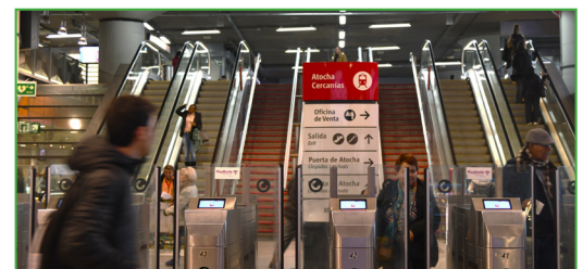
Lifts, Escalators & Lighting
